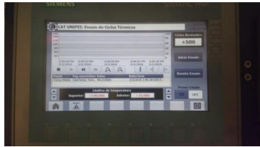
Figure 9. HMI interface screen.
