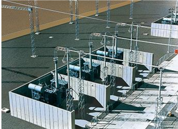
Figure 34 - Example of single-phase shunt reactor [31].
