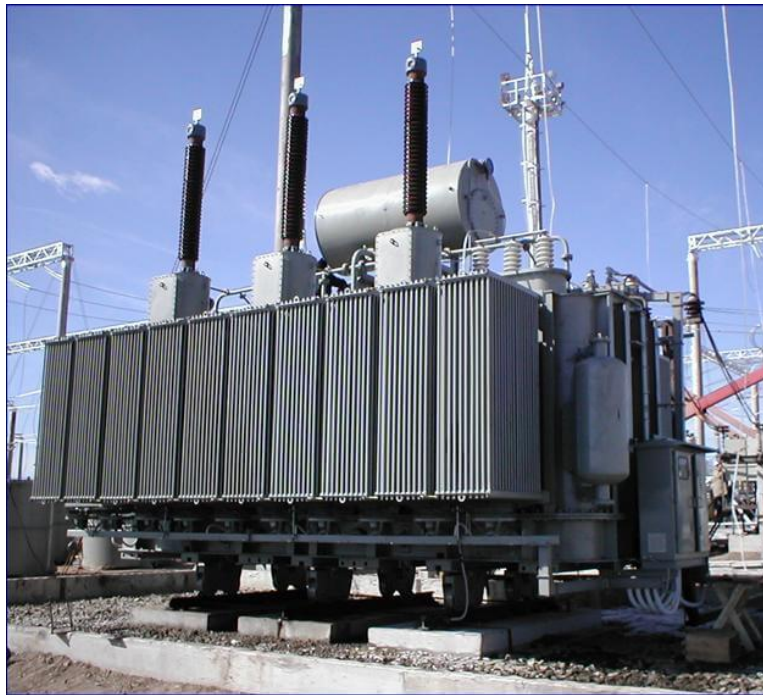
Figure 33 - Example of three-phase shunt reactor [34].
