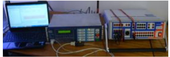
Figure 3 Test system based on OMICRON test equipment.
